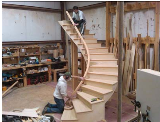
This photo shows a curved stair being fitted with a custom bent railing.
