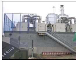
Cisterns to collect rain water sit atop the co-generational gas turbine plant as part of the “green” building efforts of the Thruway Authority.
